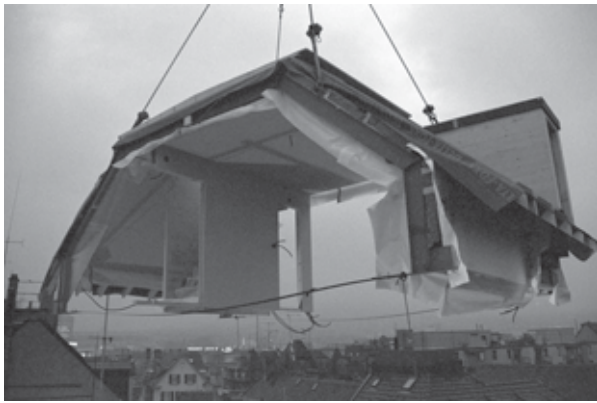
Figure 11: Pre-fabricated roof constructions offer a great potential for optimised insulation and solar system integration (Photo: Nina Mann)
